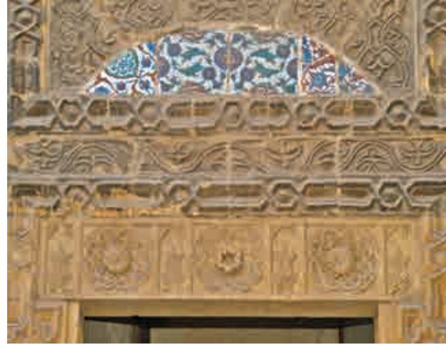
(Picture 27) The seat entrance block, stone etchings and the faience tiles, details
