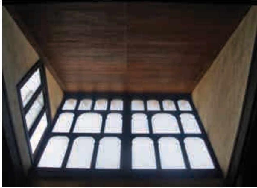
(Picture 70) The wooden ventilation daylight that covers the area in front of the grand hall
