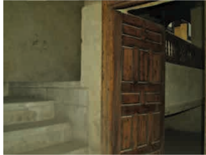
(Picture 63) The secret door (the passageway) that connects the Harem hall and the grand hall from the side of the Harem hall
