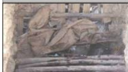
Fig. 2. Poor and unsafe latrine floors in schools
