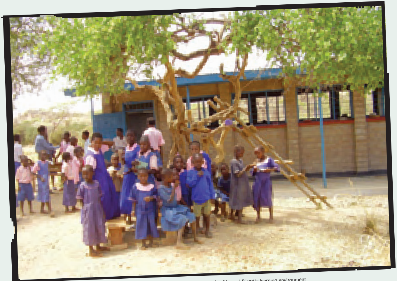
Pre-school classroom construction by local communities supported by Plan Kenya to create a healthy and friendly learning environment
