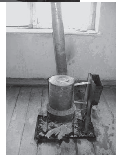
These kerosene burners are used to heat the class rooms in Hayanist school, spewing black smoke in the class rooms, and hardly providing sufficient warmth.
