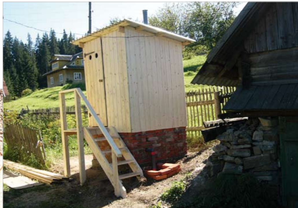
Figure 52: In total 5 of these ecosan toilets for private households were built
