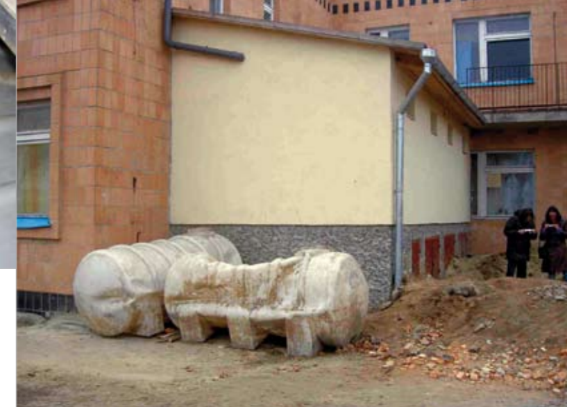
Figure 31: The urine tanks of the ecosan toilets had to be taken out of the ground again: they were not able to withstand the soil pressure
