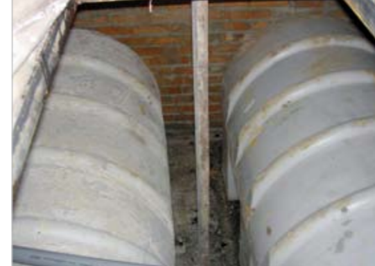
Figure 30: New urine reservoirs were placed in an underground room with brick walls
