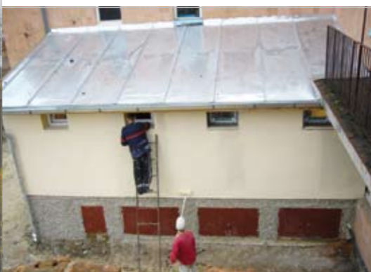
Figure 27: Through the brown doors one can access and empty out the faeces chambers
