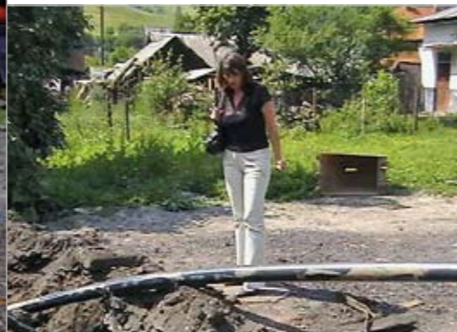
Figure 44: An additional 265 m long pipeline was needed, a branch of the central water supply system, was built, connecting more than 100 people
