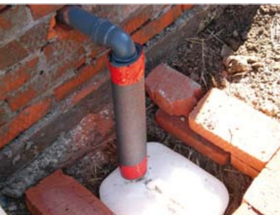
Figure 53: The urine of the ecosan toilet users is collected in a reservoir and reused on the fields
