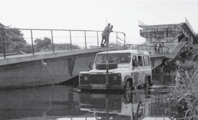
UNOHAC trying to cross the water next to a destroyed bridge over the Luaua river in Sofala province, 1993 (George Siemensma)
