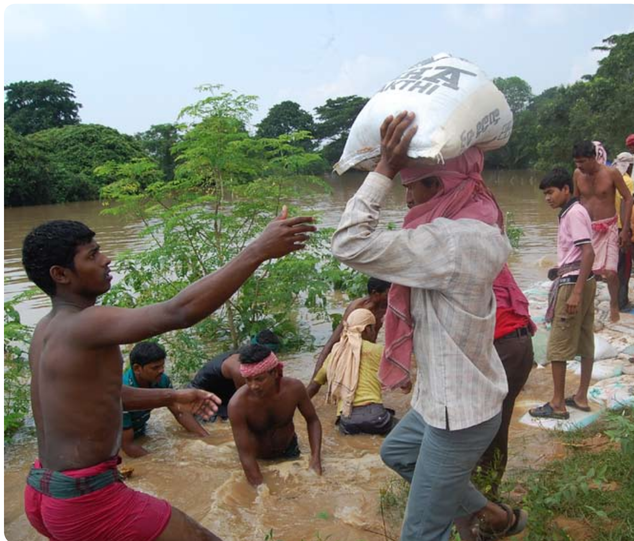
India: The local inhabitants of Orissa repairing the dikes after the flood.
