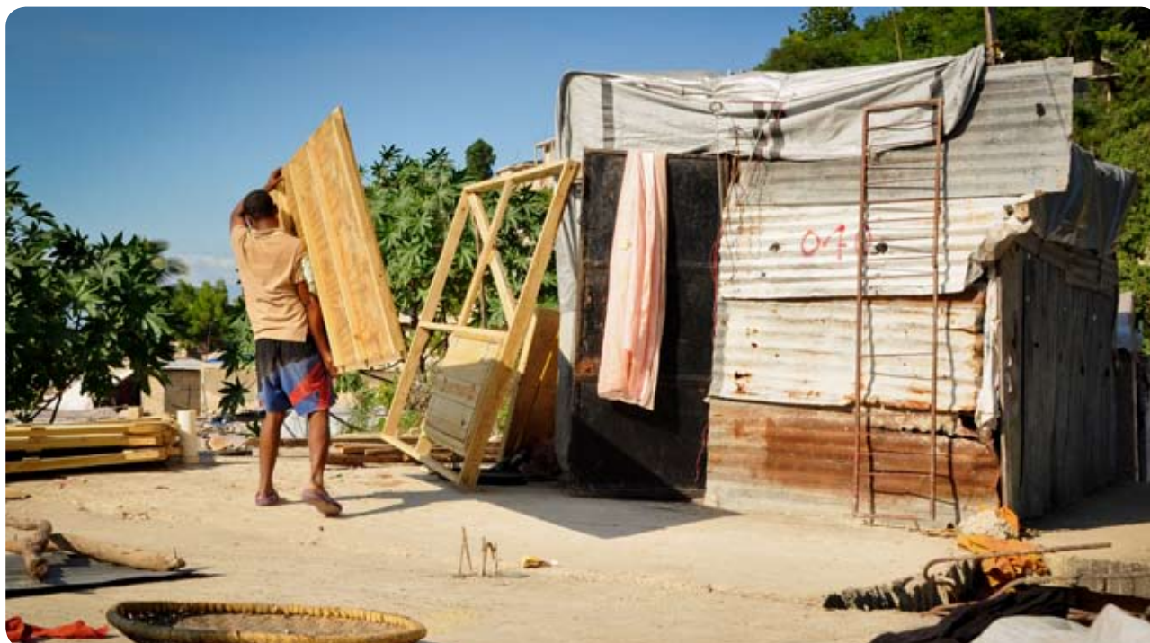
Haiti: After the emergency relief phase, Cordaid is now working on long-term reconstruction.
