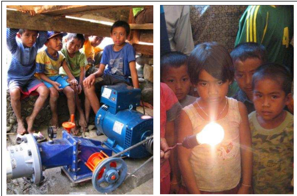
Low-cost pico hydropower as installed in Sulawesi.
