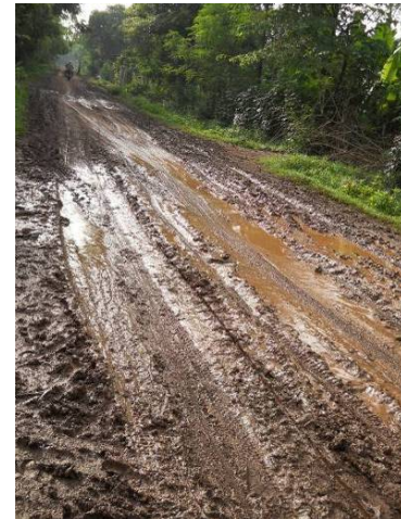
Figure 7 Road condition in Village B after rain
