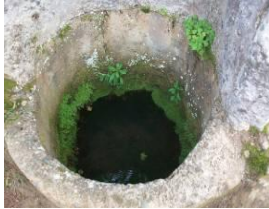
Photo: Example of a bad-maintained well
